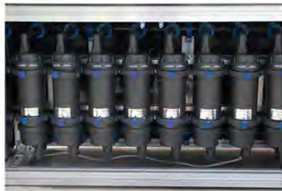
Water circulation is designed for maximum purification effect.
